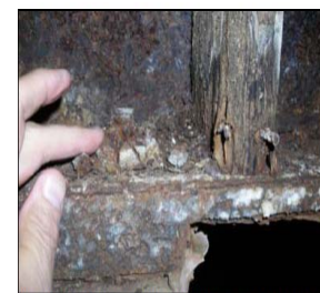
A severely rusted beam with a structural bolt that basically disintegrated in the inspectors hands
