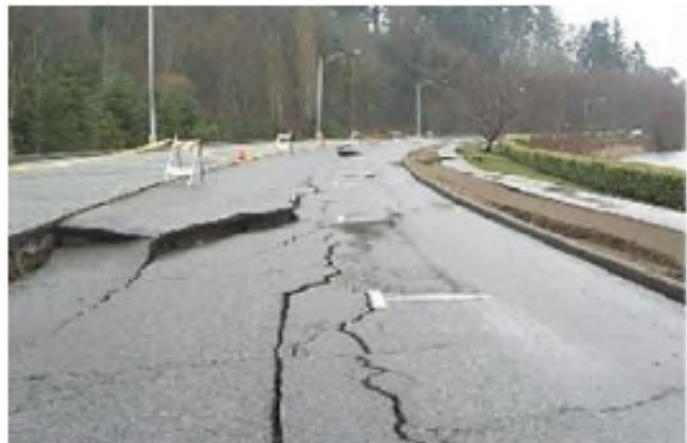
Figure 14. Lateral Spreading Along North Deschutes Parkway in Thurston County, March 2001
