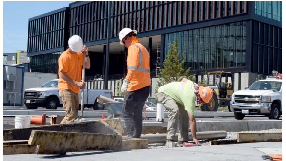
Workers build a sidewalk for Northeast Spring Boulevard, a new street in BelRed; REI's new headquarters stands behind them.
