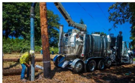
In 2016, we coordinated with Olympic on the work plan and safe construction practices to replace two poles in Newcastle.
