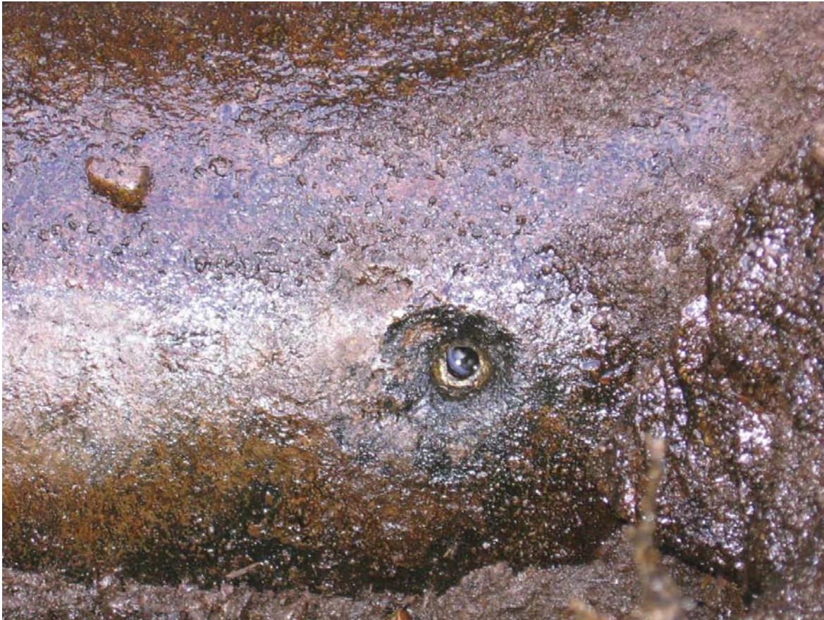
Figure 5.5.1-1 Photograph from PHMSA report showing hole in pipe wall caused by electrical fault.
