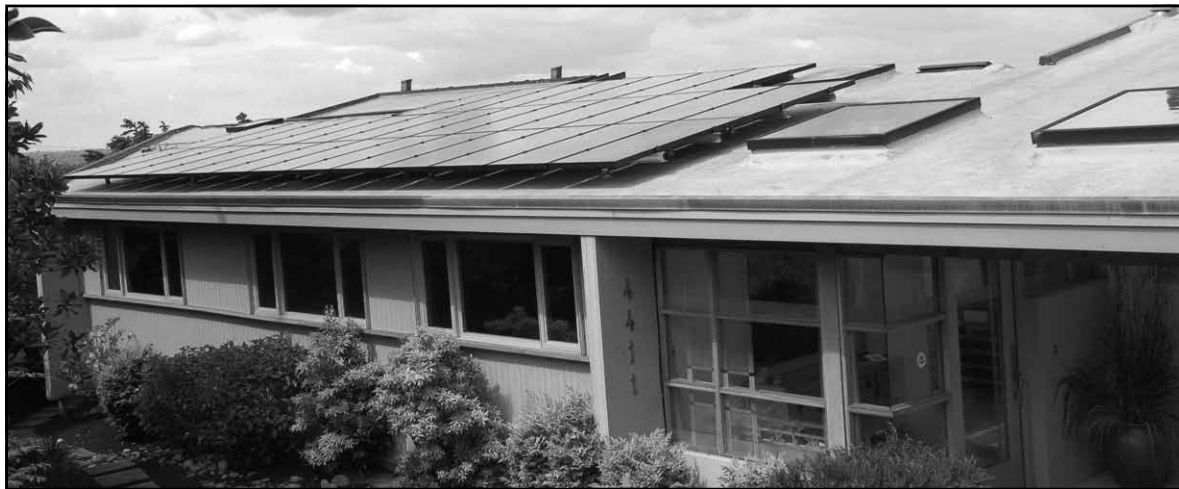
Who says the sun doesn't shine in Bellevue? The solar array on Don and Ruth Marsh's house generates electricity.
