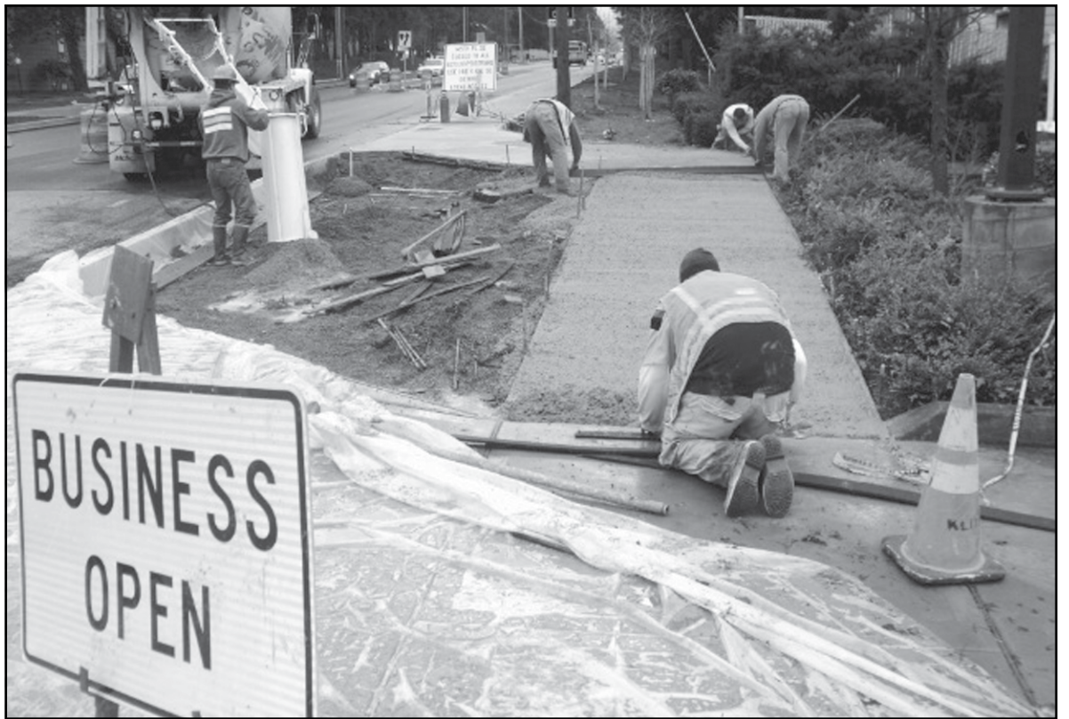
Workers install a rain garden and pervious sidewalk as part of the 145th Place Southeast makeover.
