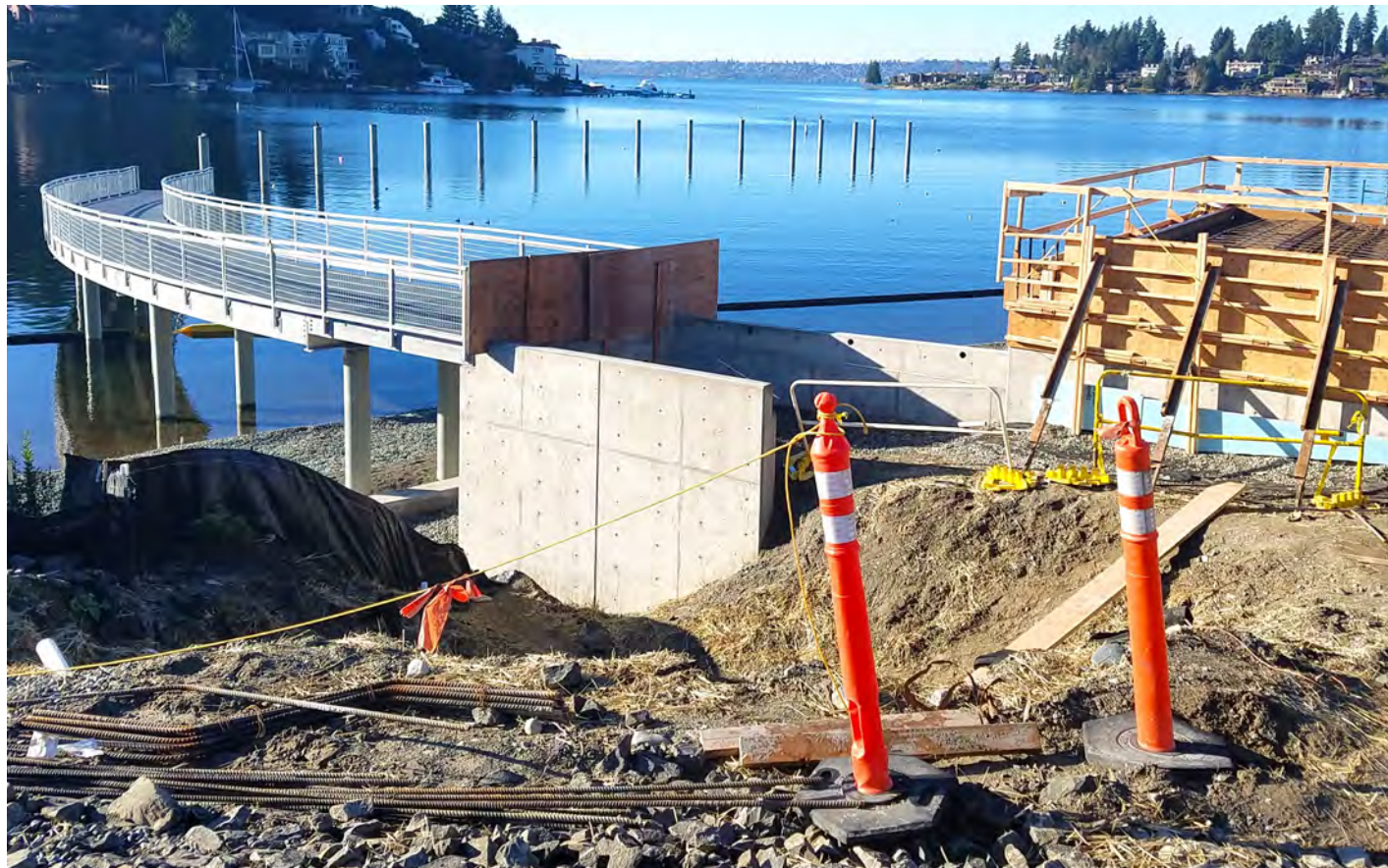
View of the curvilinear pedestrian pier under construction, with a portion of the beach house to the right.
